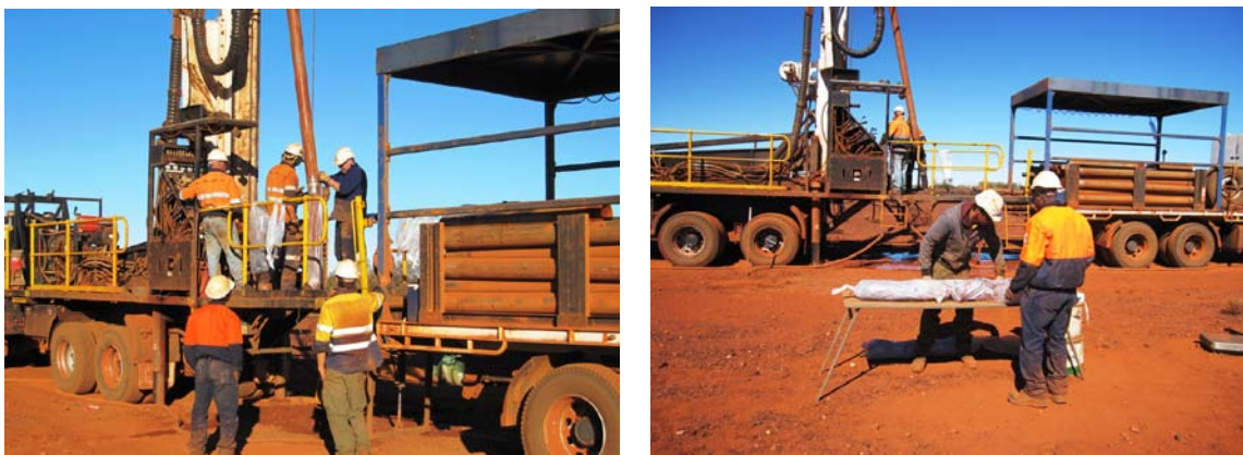
Figure 6 – Photos of Sonic drill rig showing collecting, laying out and measuring large diameter sample
